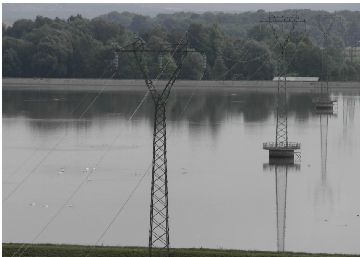
Figure 1: 110 kV Overhead line crossing Ptuj Lake with swans on the surface and other birds sitting on the second tower (Elektro-Slovenija, d. o. o., 2012)
