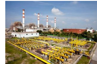
Source: Picture by EGAT via http://www.egat.co.th/
