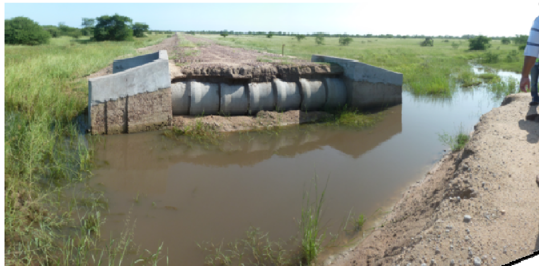
Gaza, Mozambique: road disappeared in a flood event
