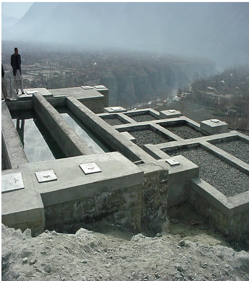
Wastewater treatment at Aliabad
